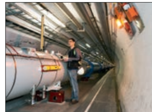
Nedo products in use at CERN
